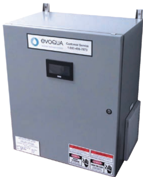
CAPAC system power supply controller (PSC)
