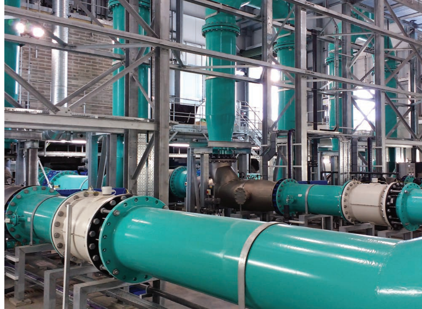
UVLX-30800-30 low pressure amalgam system in situ operating at a UK drinking water plant
